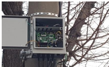
Cable TV Station
